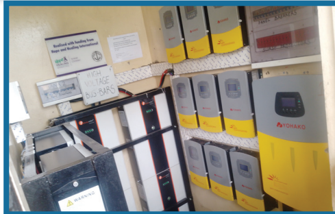
Solar panels control room
